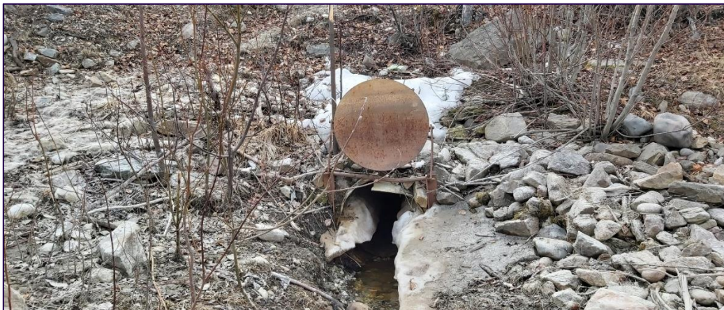
FIGURE 6.2.1. STORM DRAIN OUTLET AND VALVE OBSTRUCTED BY ICE AND DEBRIS (QUEEN STREET DRAIN).
