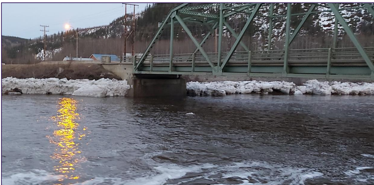
FIGURE 6.8.1. INTERFERENCE OF THE KLONDIKE HIGHWAY BRIDGE ABUTMENT DURING 2021 BREAKUP (LEFT BANK, UPSTREAM SIDE). ICE FLOES COULD ALMOST REACH THE LOWER PART OF THE BRIDGE STRUCTURE AT BREAKUP DESPITE AN ONLY MODERATE INTENSITY EVENT.
